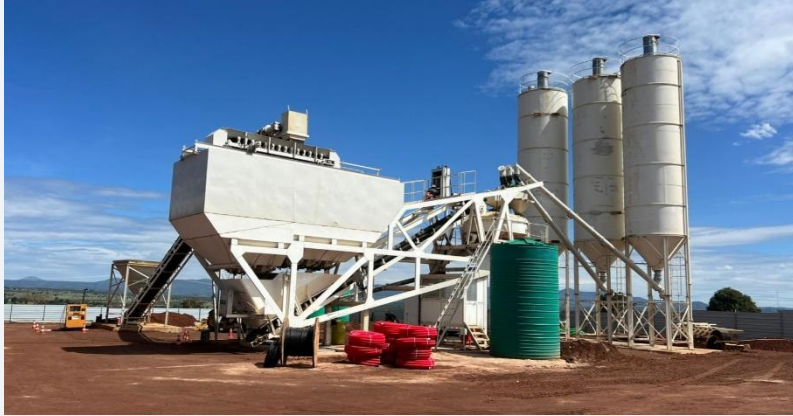
Concrete Batching Plant commissioned
